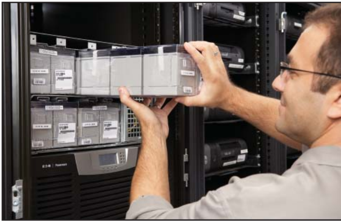
IT staff can easily replace battery modules.
