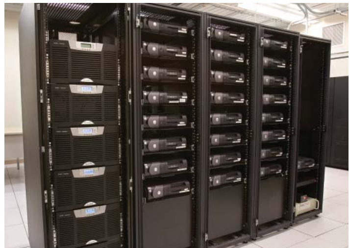
The BladeUPS remains cool even in a data center full of servers.
