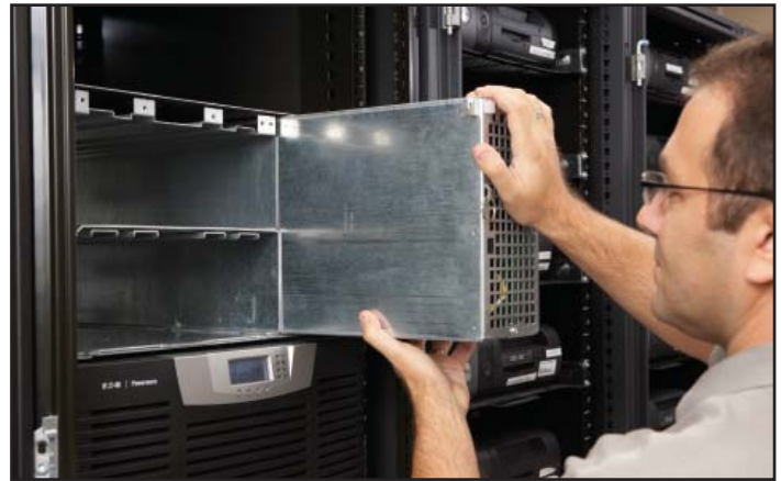
IT staff can easily install electronics modules.
