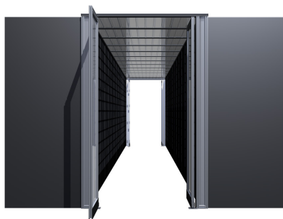
Cold aisle With Shrink-Away Ceiling and Pivot Doors
